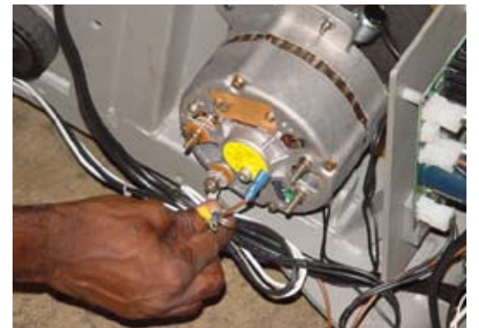
Figure 23 - Detach all cables from alternator
