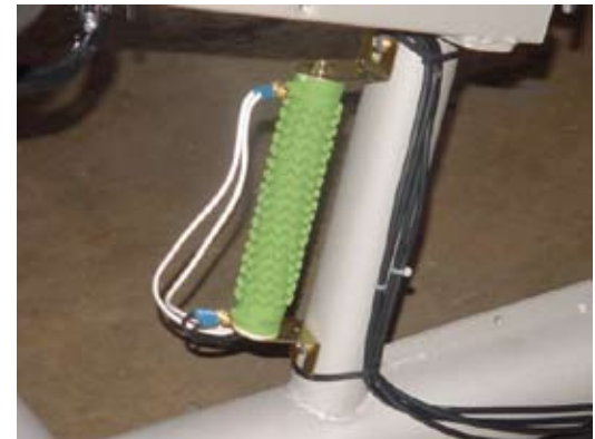
Figure 9b - Resistor wires (R916)
